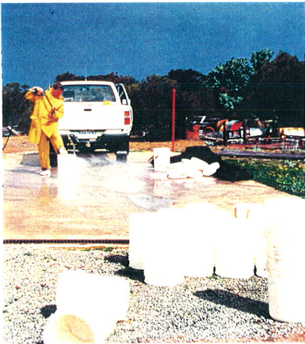
Plate 1: Equipment was washed down before installment to eliminate the possibility of spreading dieback disease. ( Phytophthora cinnamomi )
