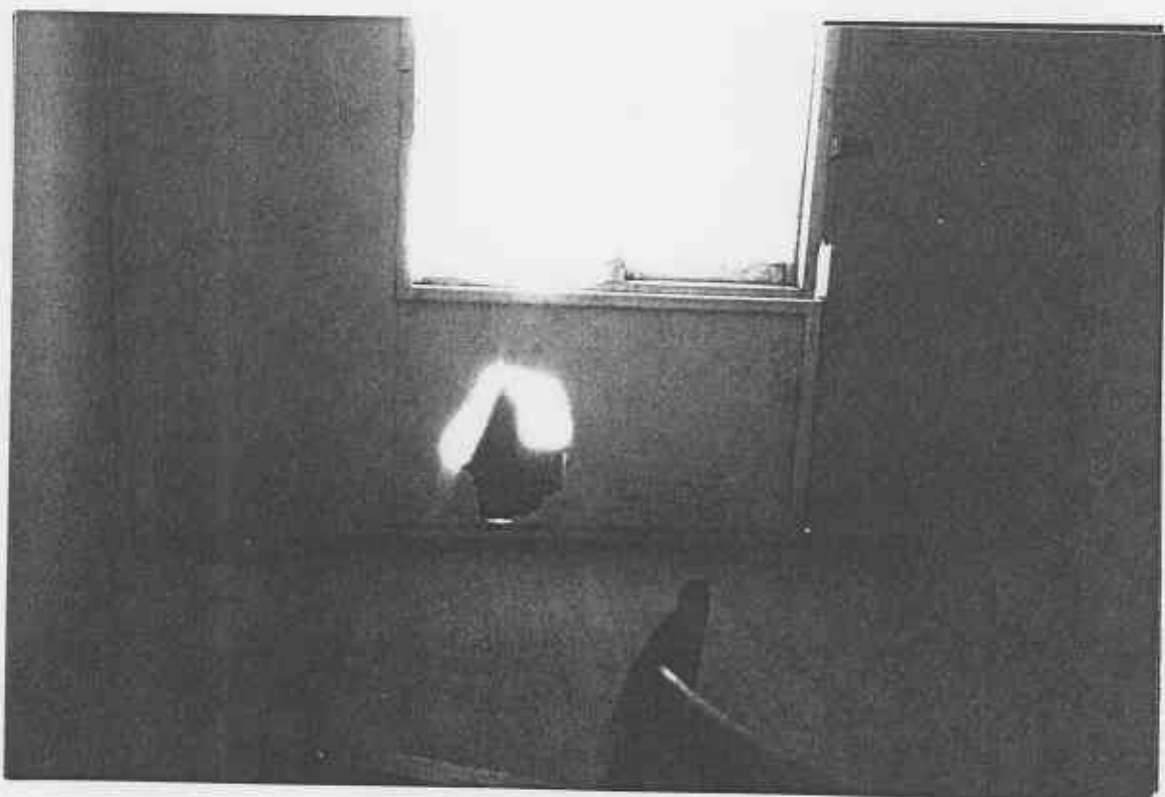
10.1.36 Many of the asbestos wall panels are cracked, damaged and broken. In this instance there is a hole right through the wall.
