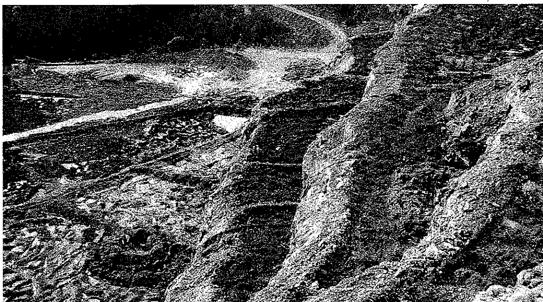
This recent example of quarry restoration in progress at Ida Bay, Tasmania, shows the attention being given to maintaining water quality. (photo D. Gillieson)
