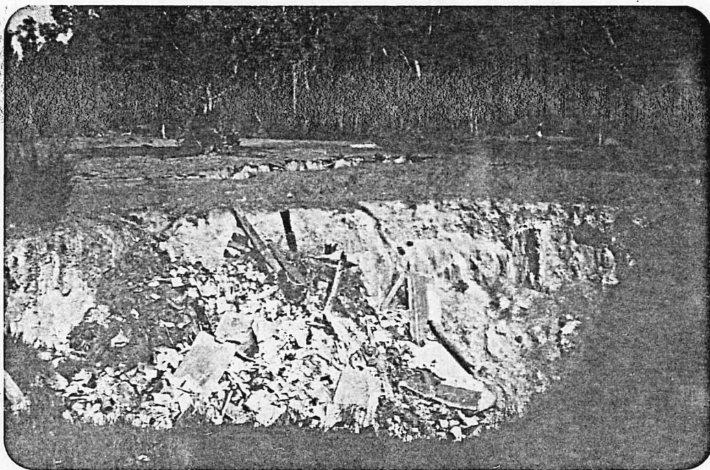
Cardiff-Neath Numerous collapses in sandy soil south of mine headquarters. This is one of the larger collapses and has been used as a rubbish dump.
