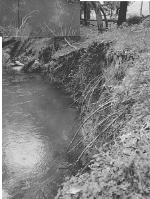
Plate 4: Subsidence or slumping of the river bank.
