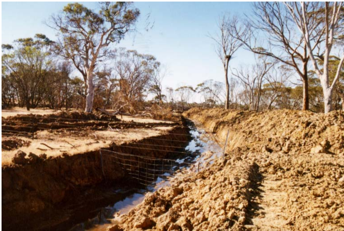
Erosion (Drain Design)
