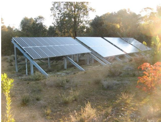
Figure 8: Current Solar Array (Photo: Elise Pinto, 2011)
