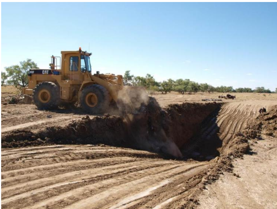
Figure 11. Burying Cylindropuntia fulgida near Longreach, Queensland, using a front end loader (photo from Desert Channels Queensland).
