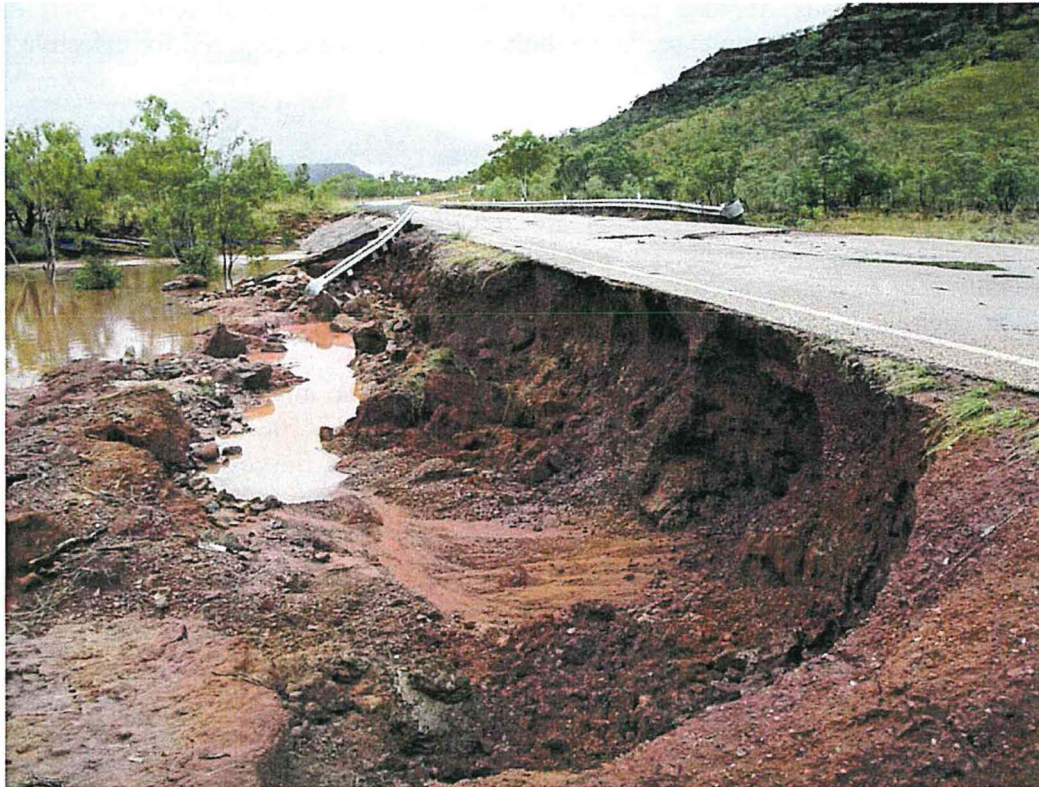
Fig. 3. Flood damage to the Victoria Highway, NT, in April 2006.
