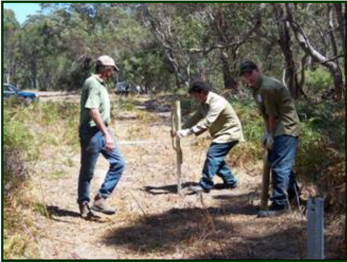
John Dennis with Green Corps erecting a fence to protect the Hay River
