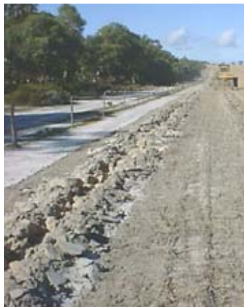
Figure 1. The presentation of a rip line following ripping with a single tynd dozer ripper to a depth of 70 cm. The central part of the rip line is like a trench. Subsoil boulders are lifted to the surface by the deep ripping and the angle of the tyne digging tip.
