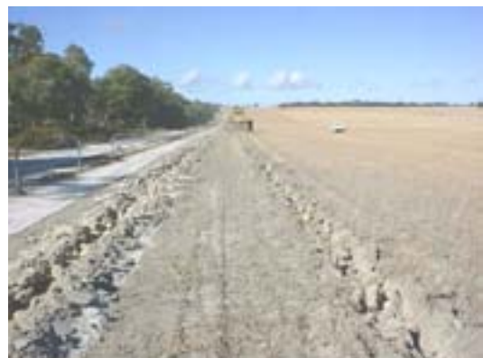
Figure 4. Deep ripping with a dozer dilutes the topsoil. Subsoil boulders and loose subsoil particles are lifted to the surface in the centre of the rip line. A combination of ripping implement design and predetermined ripping depth can greatly minimise topsoil dilution.
