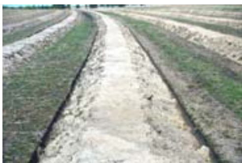
Figure 9. A well constructed mound showing best-practice 'flat and smooth top'. A wider ripping width prior to moundploughing facilitates improved mound construction and also lessens wear and tear on the moundplough.
