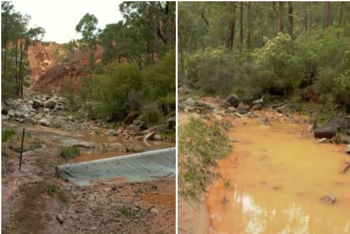
Figure 49. Photographs showing the dam work and increased sedimentation and turbidity in the stream below Stirling Dam (HAR20) in 2007.
