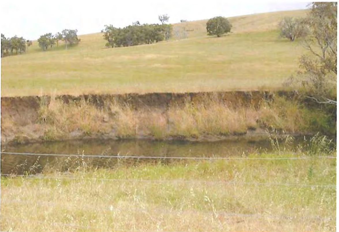
D2 Grade Foreshore: The channel has eroded away over time, leaving a weed (mainly annual grasses) infested drain. No native vegetation occurs at all on these banks.
