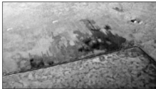
Leaking channels have been identified as an important source of water loss from a conveyance or distribution system.
