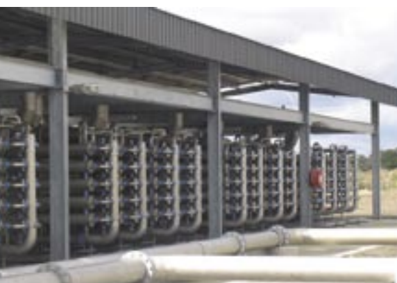
Figure 7 Membrane filtration bank for recycling water at South East Melbourne
