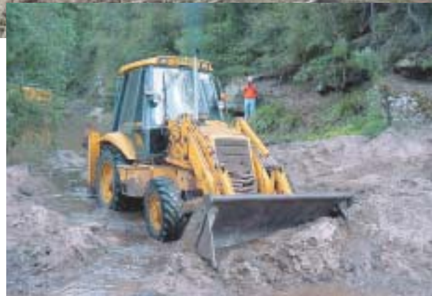
Photo 39. A 4WD tractor/loader like this one is an essential piece of equipment at a log structure construction site. It can be used for moving logs around on site, backfilling structures and regrading the site.
