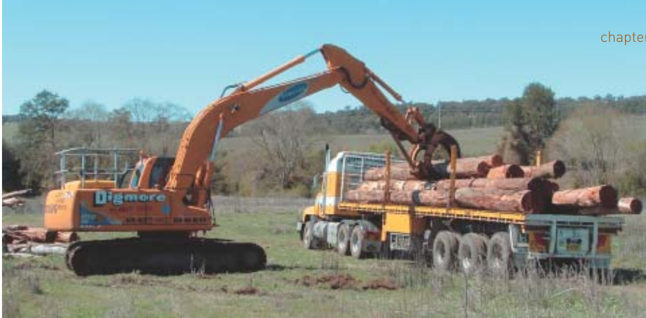
Photo 42. A 22 tonne excavator with a non-rotating grab offloading logs (without root wads) for use in bed-control structures.
