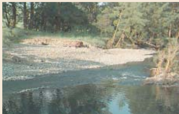
Photo 35. Bank deflector jam that appears to have failed, but in fact is still there — only buried. This is a case of the structure being over designed and too effective — to the extent that it initiated so much deposition that the whole structure was buried and the channel shifted laterally by ~20 m. In this case the structure is still performing its primary engineering role — even while buried. It provides woody substrate in the hyporheic zone, and a source of slow release carbon to the system. In this instance we may need to reconsider what is meant by “failure”.
