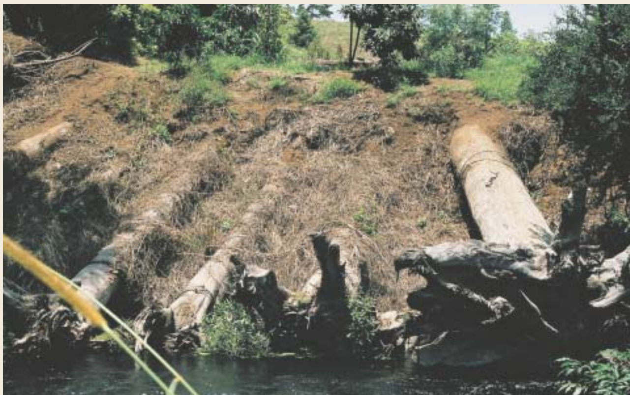
Photo 8. Early model log bank revetment, with cable and rock ballast — Obi Obi Creek, Queensland.
