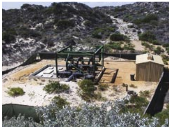
Figure 17. Cognis Pty Ltd, pumping station.
