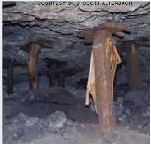
Stull buckling under increasing pressure of the ceiling settling over time.
