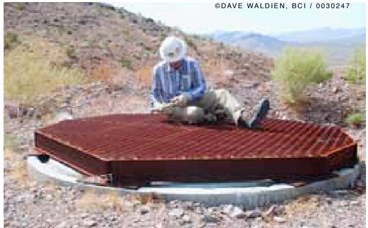
A grate is placed on a vertical culvert to maintain airflow in the mine.
