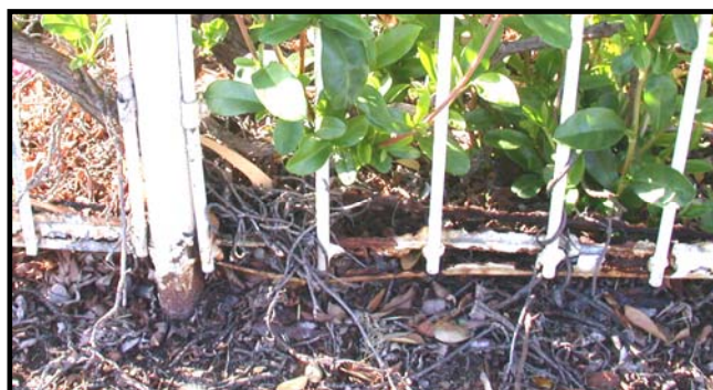
Figure 5. Corroded metal fence
