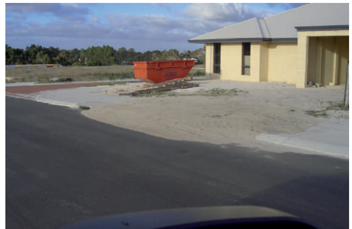
N Poorly protected site with building sand spilling onto road near storm water drain
