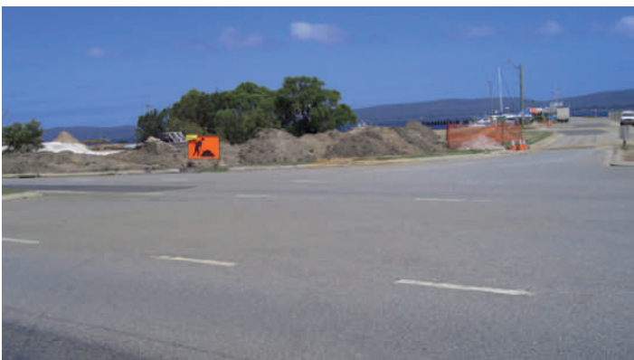
N Stockpiles with inadequate protection
