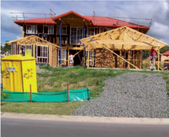
Y Sediment control fence along the lower edge of a residential building site
