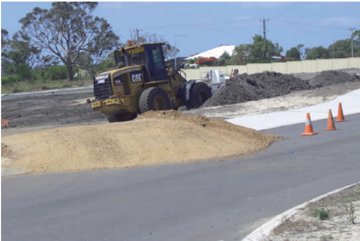
N Earthworks commenced with no sedimentation protection
