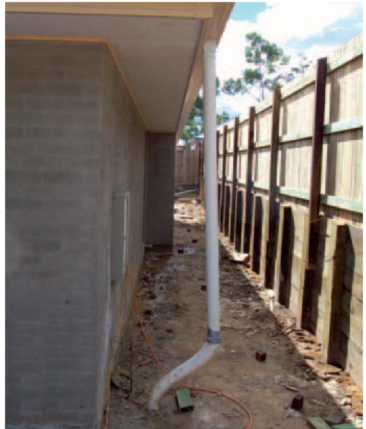
Y Temporary roof drainage
