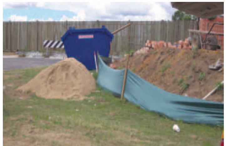
N Poor site planning – stockpile outside of sediment containment fence
