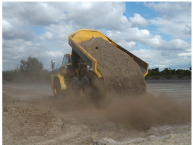
D. Topsoil spreading at Jandakot Regional Park in April 2012. Soil was spread to a uniform depth of either 5 cm or 10 cm.
