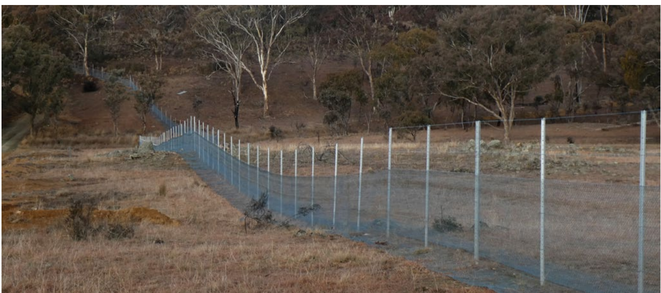
Wandiyali Restoration Trust conservation fence under construction in NSW just south of Canberra. Photo: C. Larcombe, Wandiyali Restoration Trust
