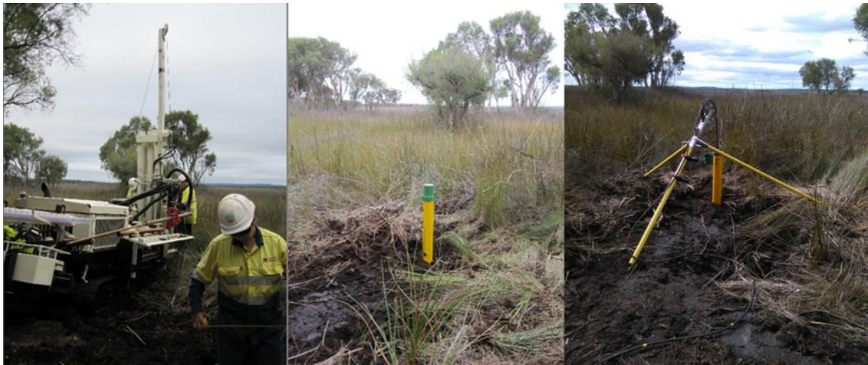
Figure 10: Geoprobe 7822DT push-probe drill rig used to construct lake shoreline bores; Byenup BY01/03 construction (left and centre) and geophysical logging with VistaClara Dart NMR tool in May 2015.
