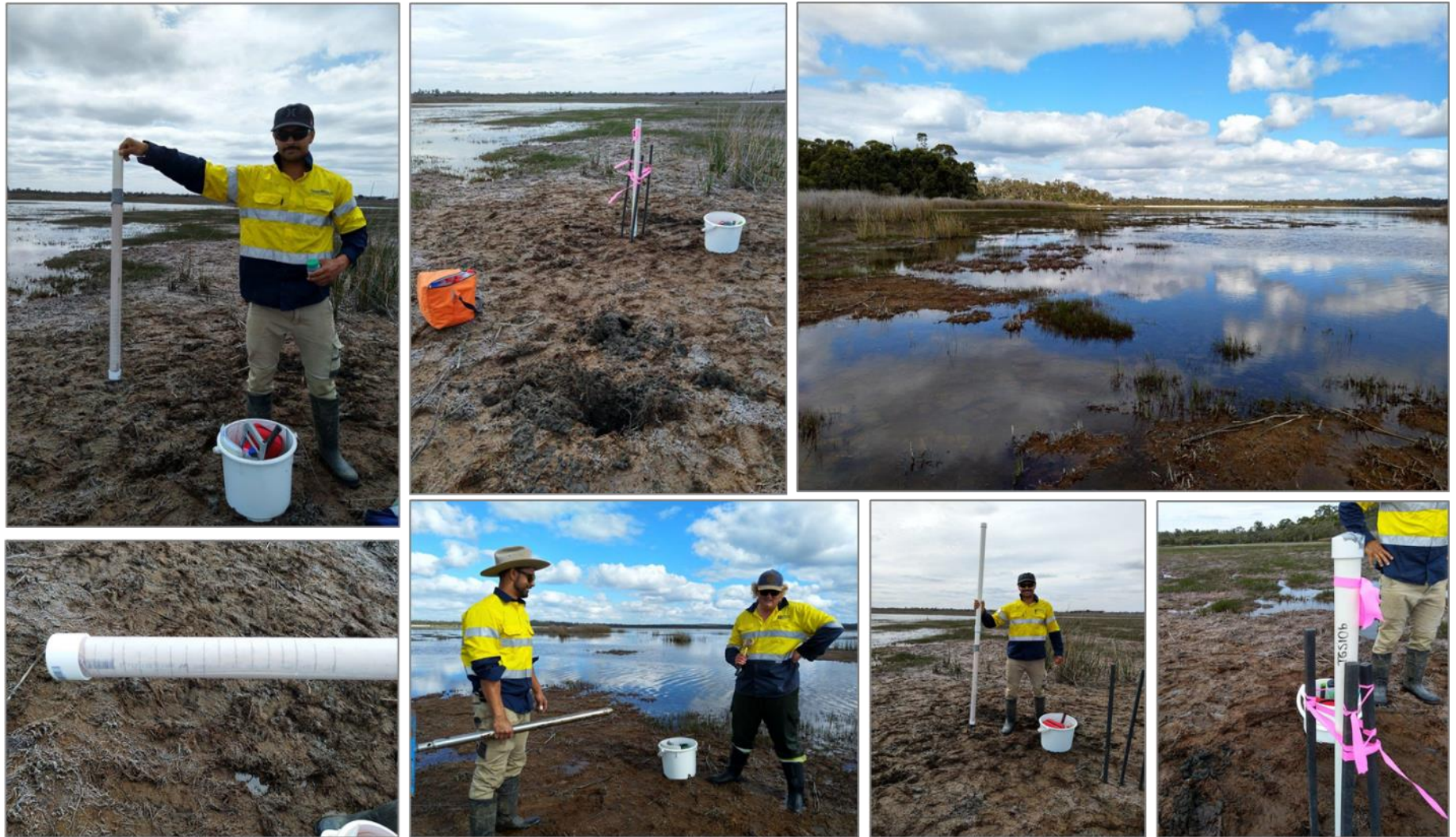
Transect 2 site TGN10b – mini piezometer construction, showing location in relation to the southern surface water body, stick-up and screen slots with filter sock
