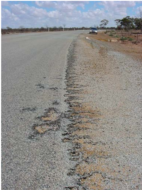
Damage to road surface
