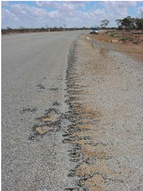
Damage to road surface
