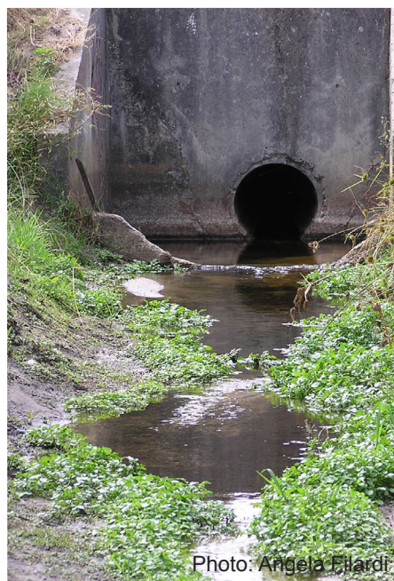
Drain in Lower Canning catchment, April 2004. Photo: Angela Filardi
