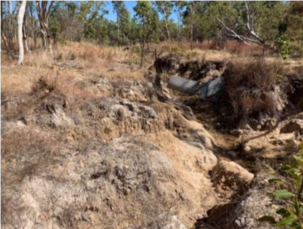
Figure 2. 2019 significant erosion at water outflow point at MtElizabeth1a/d (Middle spring) (from Chemello 2019).
