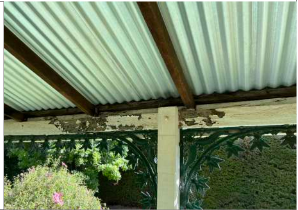
Damage and weathering to verandah beams
