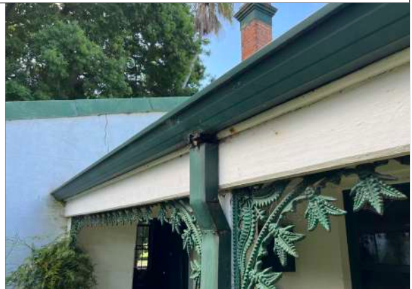
Damaged down pipes to verandah
