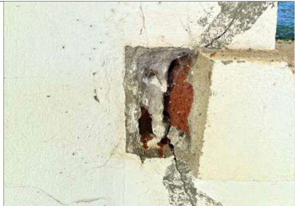
Damage to window sill (W3)
