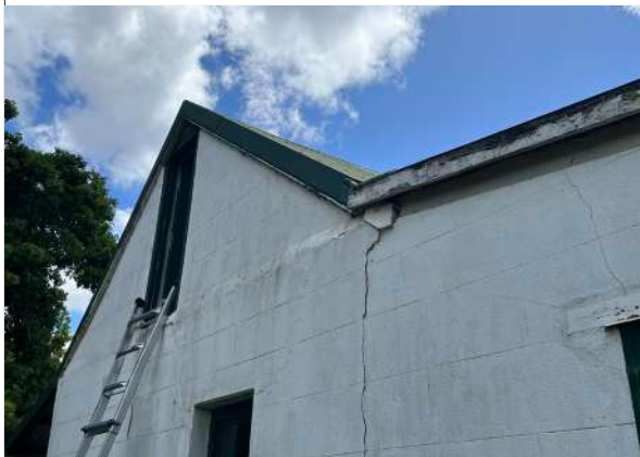
Cracking to south facade
