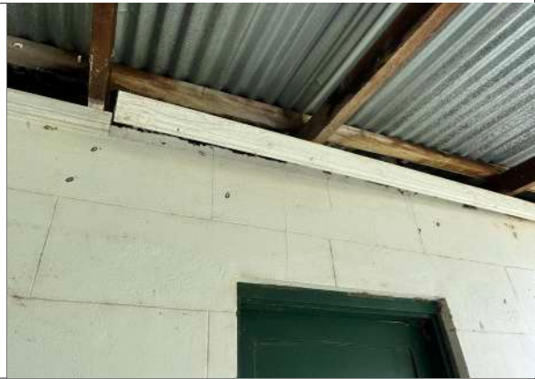
Damaged external cornice to side verandah
