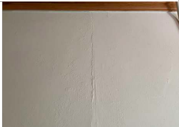
Large filled crack to Study
