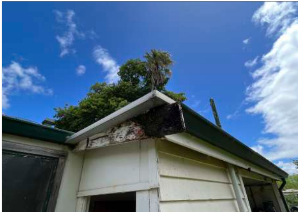
Damage to fascia above toilet
