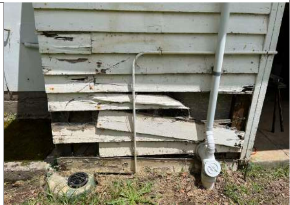
Toilet wall damage
