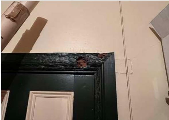
Termite damage to D8
