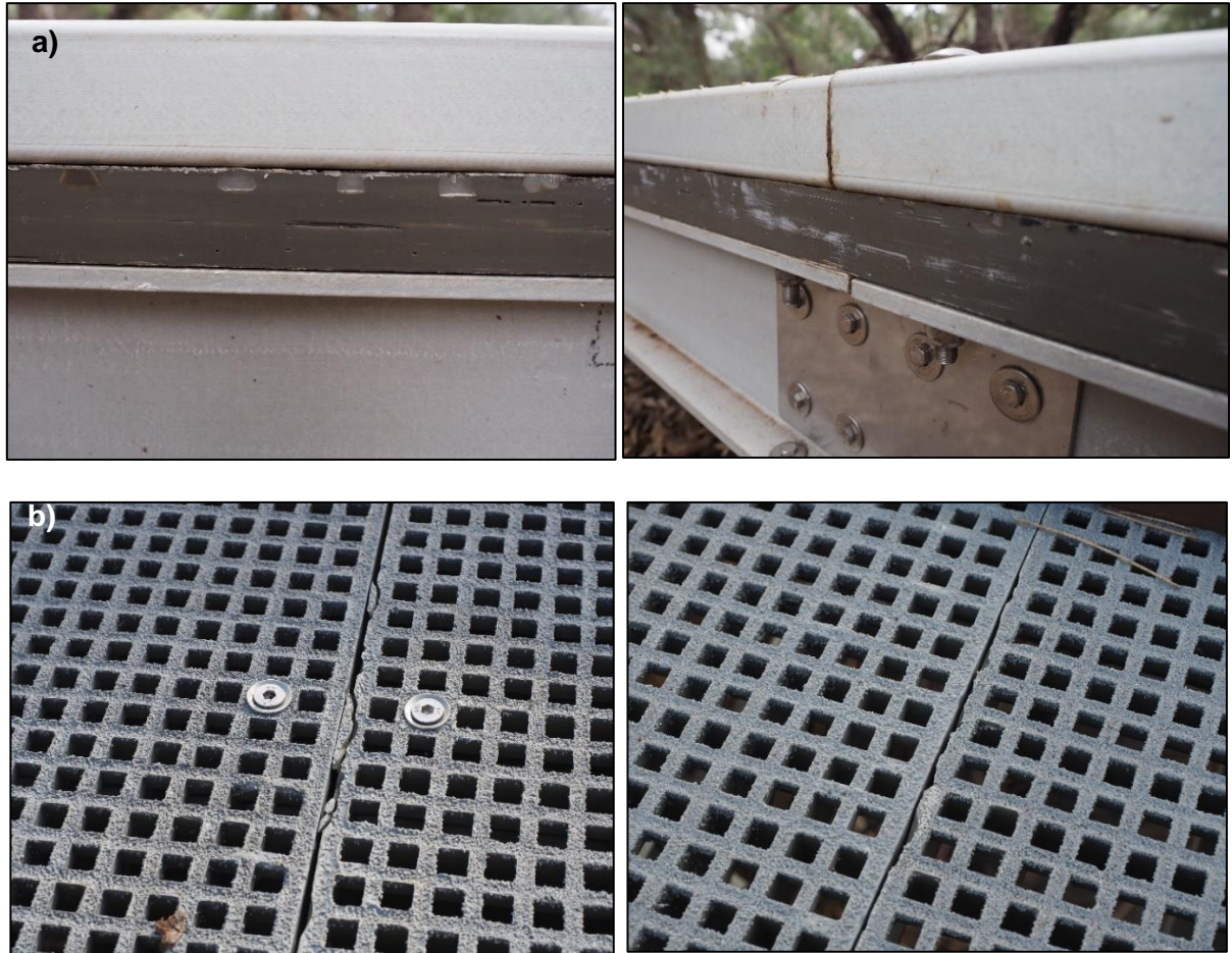
Figure 18. (a) Fibre reinforced plastic (FRP) kick rail (top), FRP mini mesh edging (middle dark grey layer) and FRP substructure (bottom layer) along board walk at Thornlie nature reserve; (b) FRP decking joints at Melville bird view platform.
