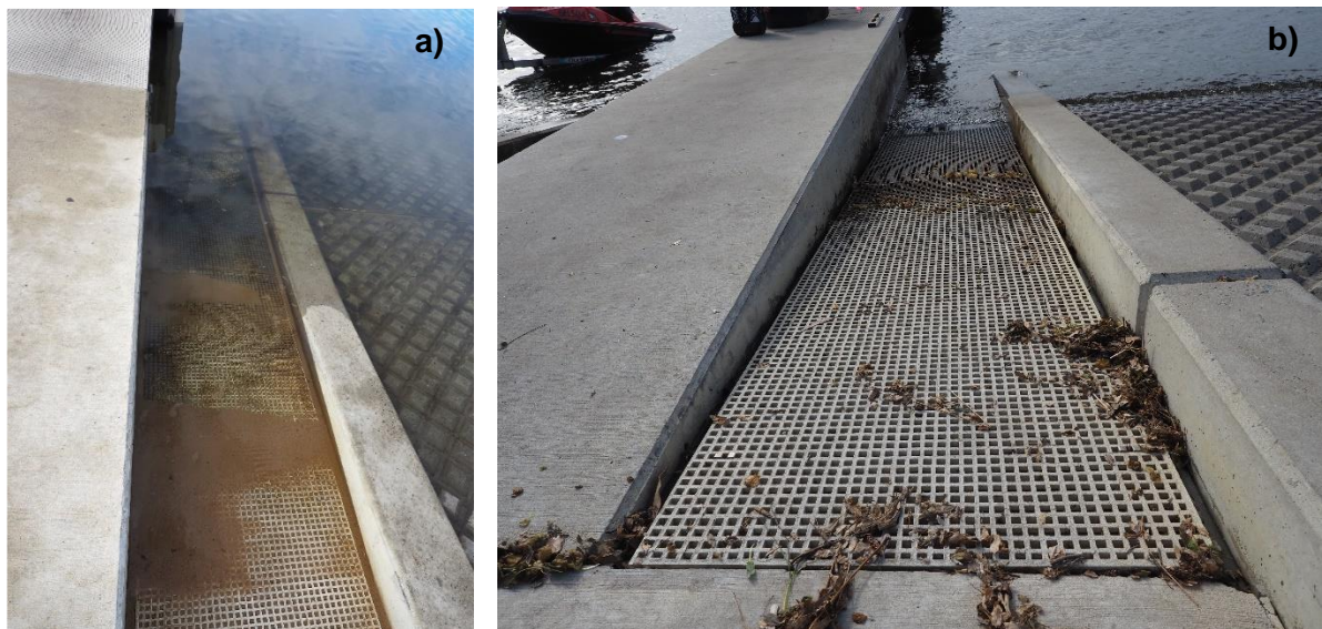
Figure 34. Examples of fibre reinforced plastic exposed to wet and dry cycling at Deep Water Point (a) and Point Walter boat ramps (b).
