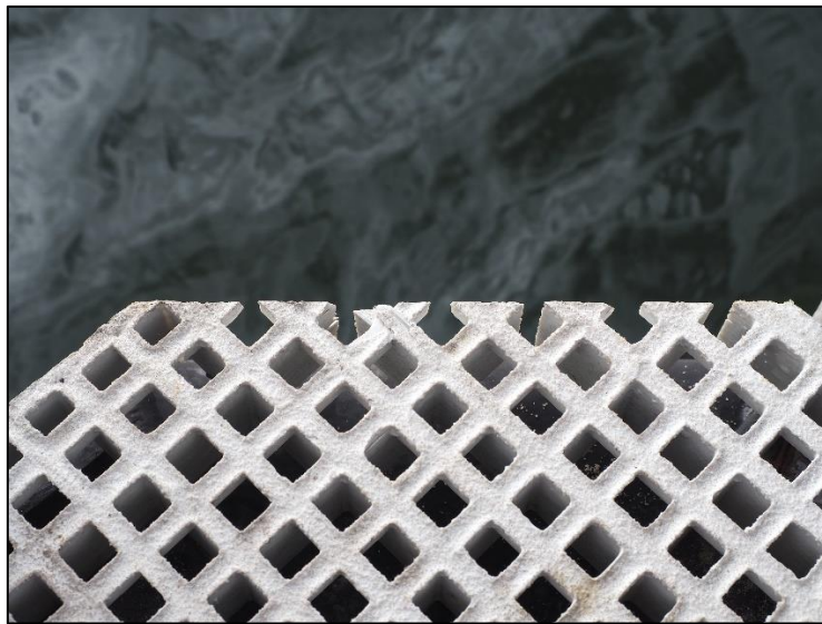
Figure 36. Fibre reinforced plastic decking cut on an angle and showing chipping at the end of Deep Water Point finger jetty.
