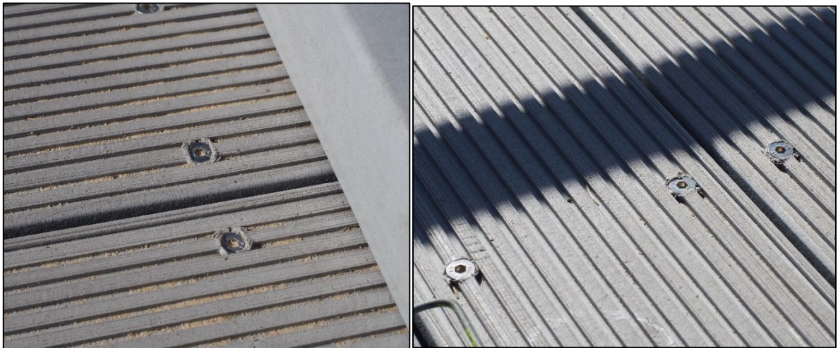
Figure 24. Poor installation of screws to install recycled plastic decking at Rockwood Street (Esplanade) jetty.
