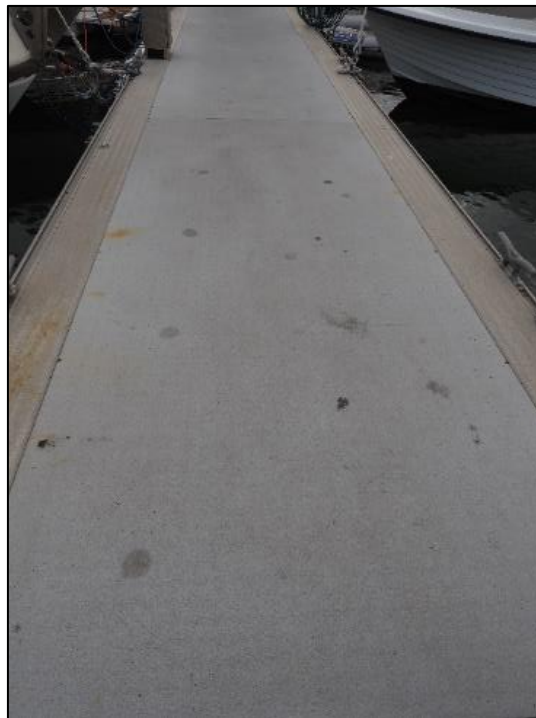
Figure 35. Staining of solid top fibre reinforced plastic decking on jetty at Swan Yacht Club.
