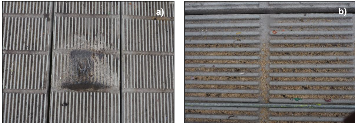
Figure 22. Material loss observed on recycled plastic decking at the Mount Henry jetty (a – chemical or fire damage, b – exposed plastics of different colours).
