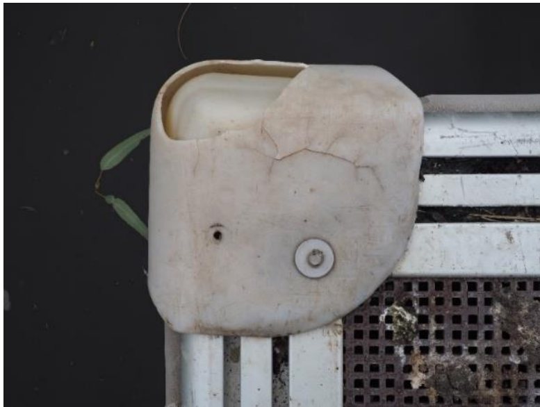
Figure 31. Damaged rigid capping used on corners of the pontoon at Middle Swan Reserve.
