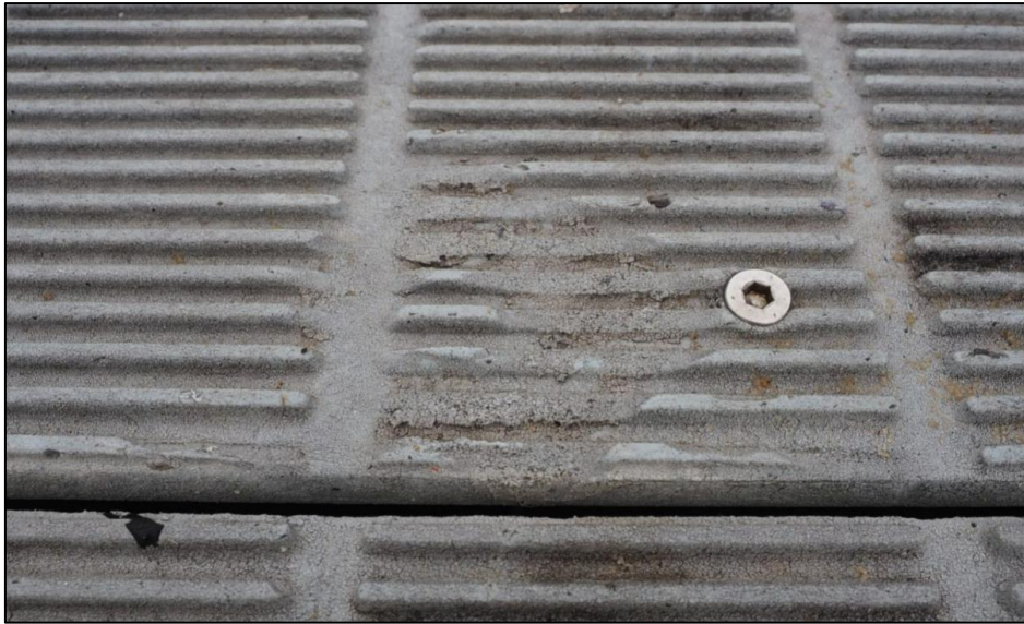
Figure 25. Correct installation of screws to install recycled plastic decking at Mt Henry Jetty.
