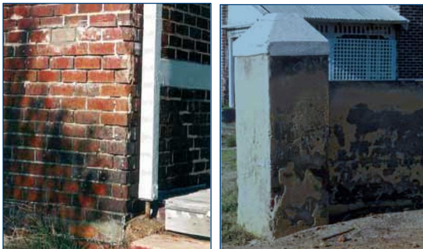
Figure 5. Examples of damage to infrastructure caused by salinity
