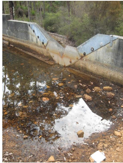
V-notch weir on More Seldom Seen Brook, down-stream of sampling site
