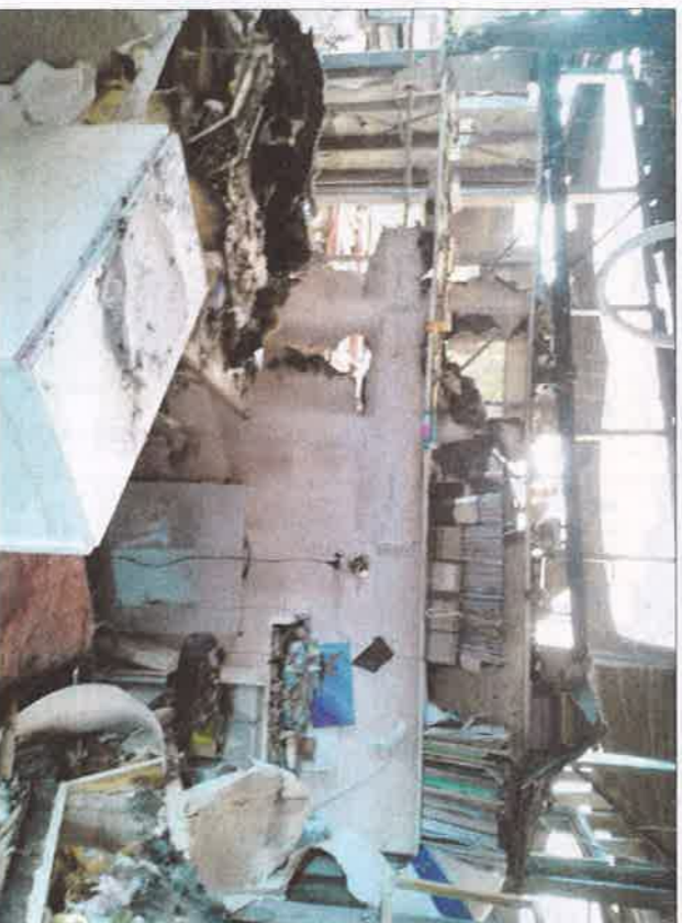
John and Elaine Wakka's garage and workshop/studio were destroyed by fire.
