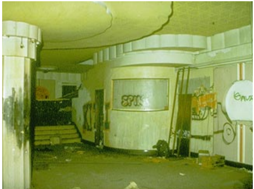
▲ Results of vandalism on the Sun Theatre foyer, Yarraville, Vic. Cultural heritage needs to be acknowledged, valued and protected.
