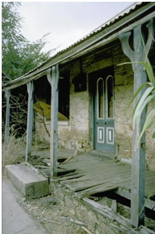
▲ Unoccupied buildings are prone to physical decay and vandalism. This cottage in Yass, New South Wales, contributes to the historic character of the town, but it has been allowed to deteriorate.
