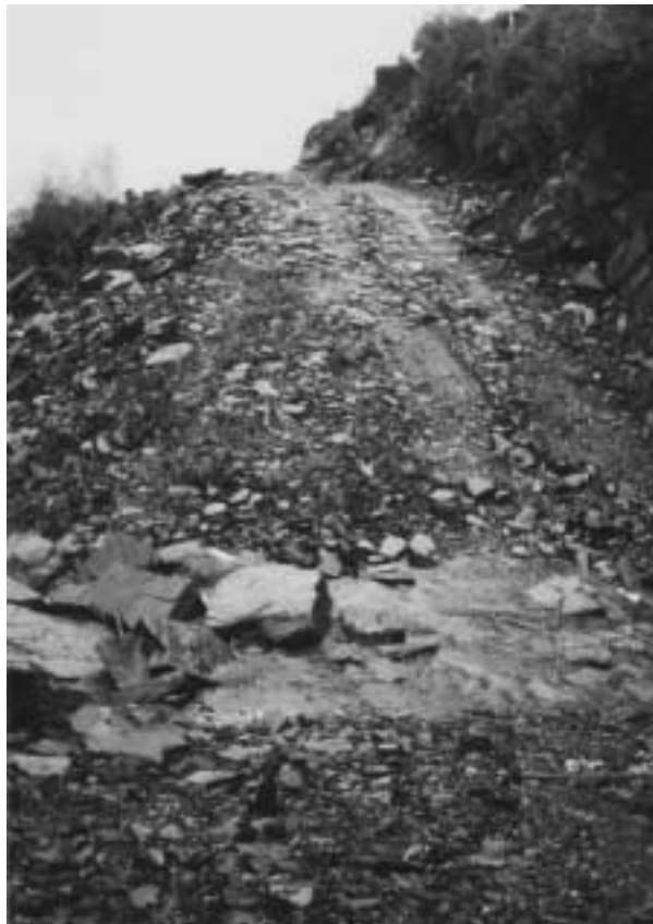
FIGURE 21 Armoured cross-drain on a semi-permanently deactivated road in the Three Arm Creek sub-basin (A. Hasanen photo).
