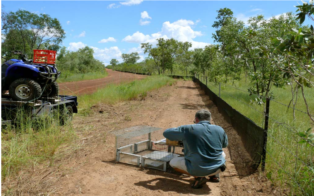
Section of fence line under construction, showing graded scrape along east side used to bury the shade cloth and a trap being prepared for deployment
