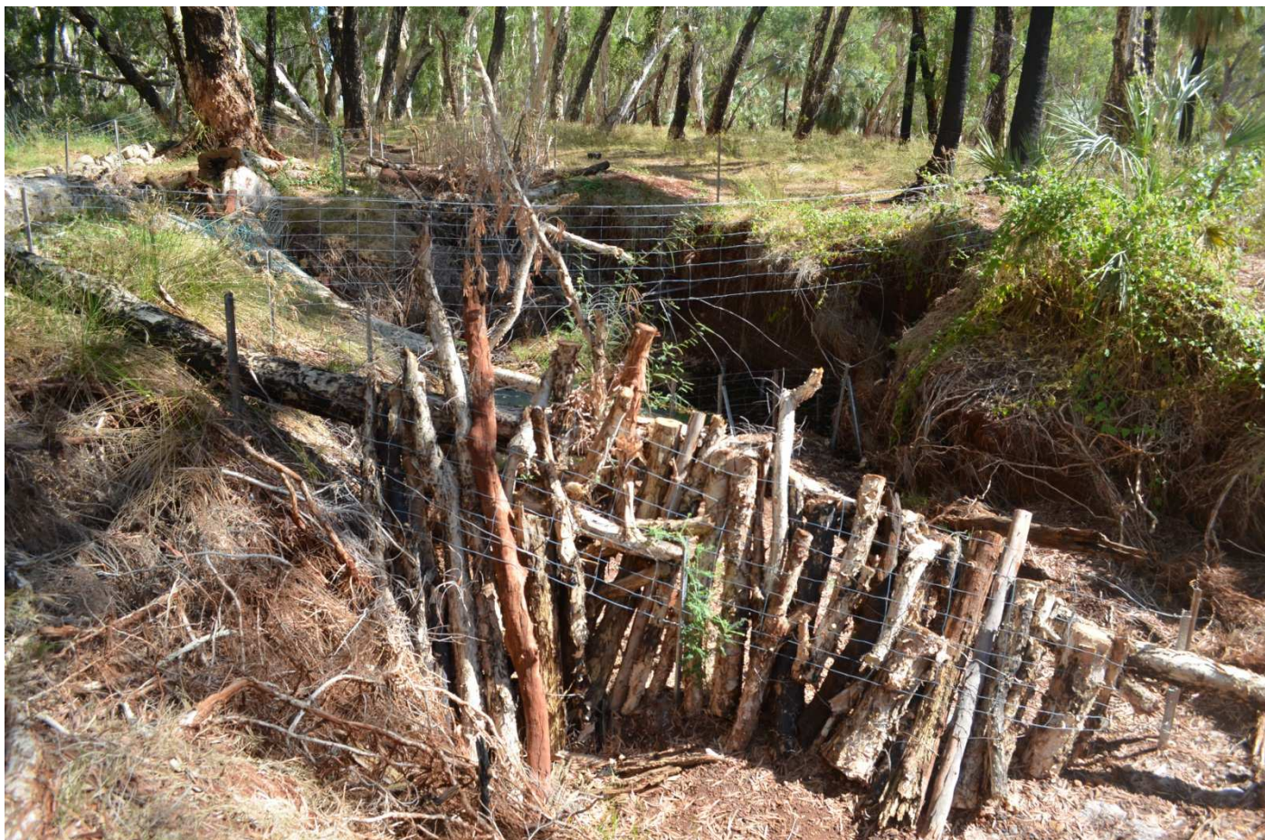
^^ Main erosion gully looking upstream toward headcut, Oct 14
