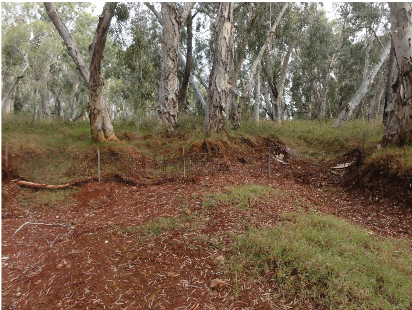
^^ Main side gully no significant change, July 15
