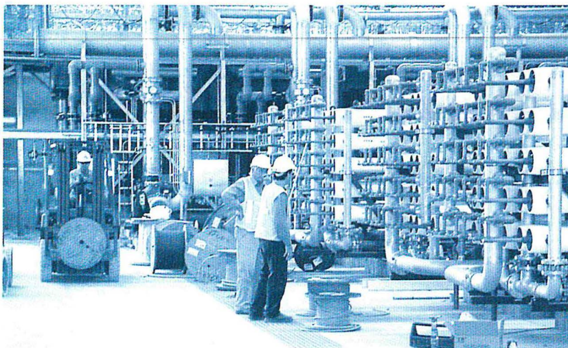
The Kwinana Water Reclamation Plant is nearing completion. It will provide highly treated wastewater to industrial customers and free up five gigalitres of scheme water for domestic use.
