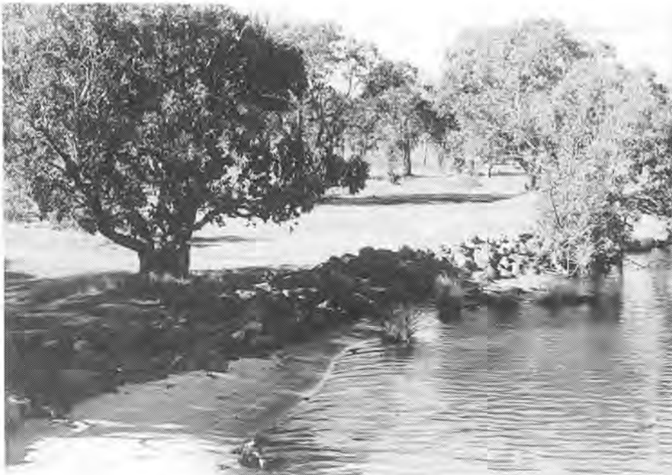
Erosion control such as rock walling is required to protect the riverbank
