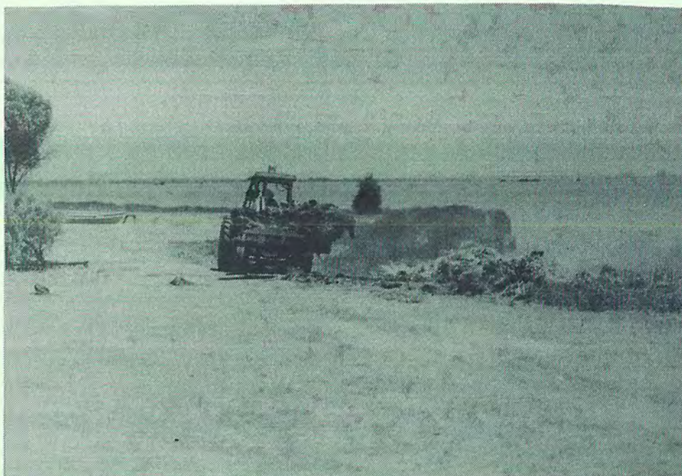
Removal of algae and rubbish is required along foreshore areas.
