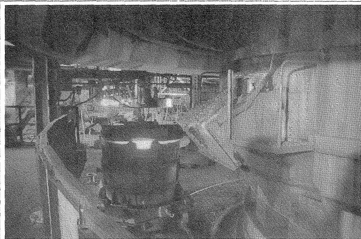
20. A ladle being pre-heated ready for tapping. Just right of centre is one of the furnace tapholes which is plugged.
