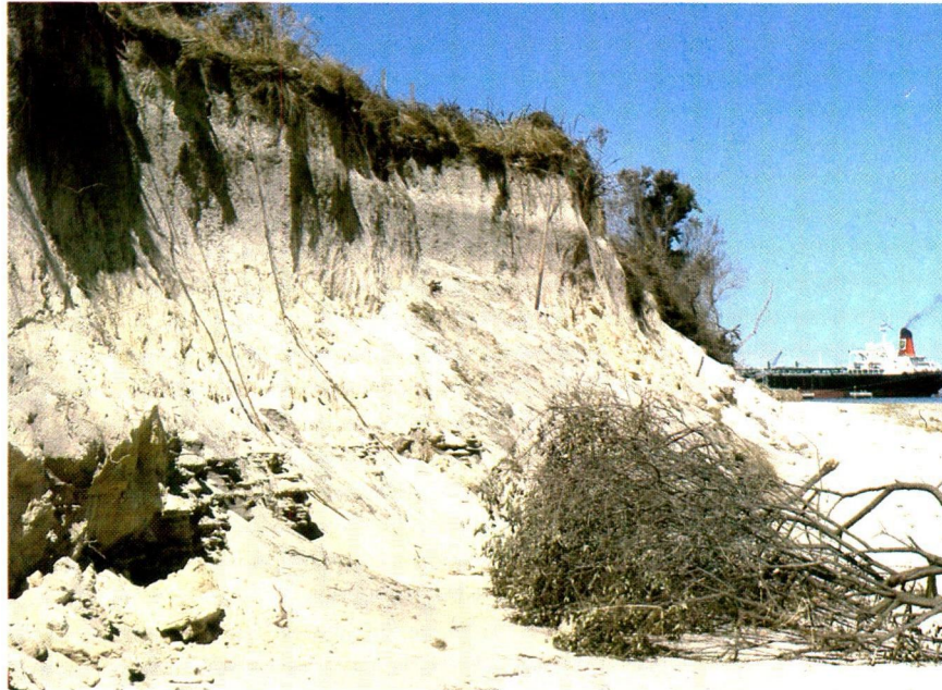
Beach erosion cutting into vegetation on the north side of James Point.
