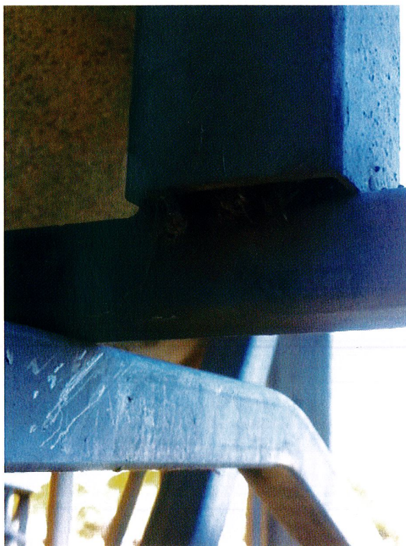
Left: The base of the tube where it rests on the cross strut. A petrified bat can be seen where it tried to squeeze out, but was unable to do so. This gap at the bottom is only 8mm x 38 mm wide. Changing the cross bar at the bottom to provide a larger gap would help with future design, but the top cap (see below) will solve the current problem. Photo: Dayle Lloyd
