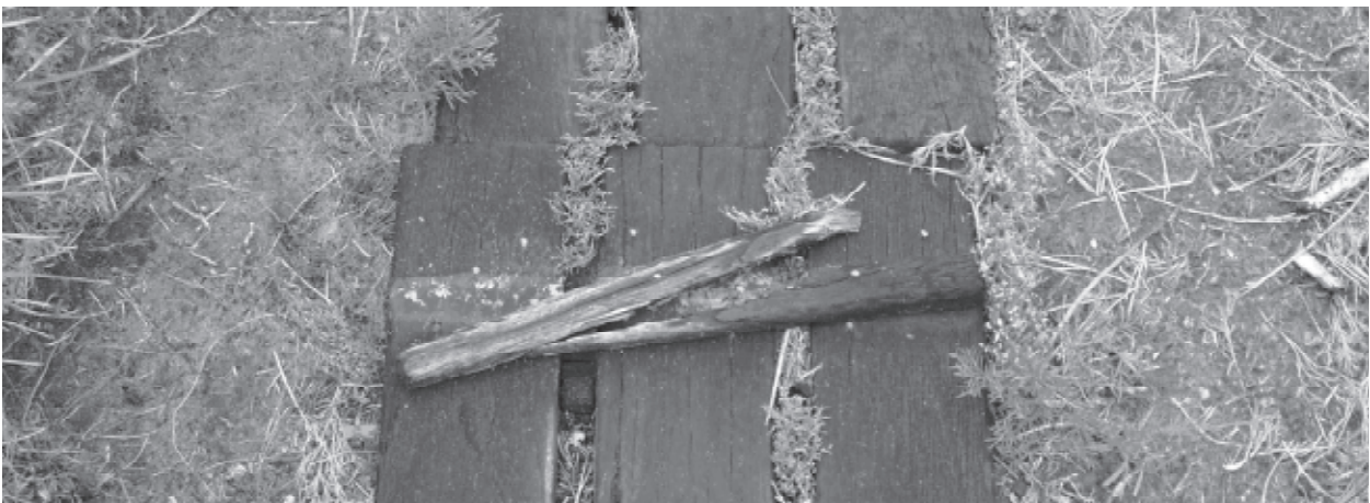
Figure 10. A charred board-walk with split cross tread and protruding nails, moderate-poor condition but moderate-excellent / excellent effectiveness rating for Bibbulmun Track in WCHNP
