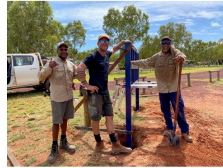
Nathan Hunter, Dane Johnson and Tony Turner installing signage at Eighty Mile Beach. Photo by DBCA.
