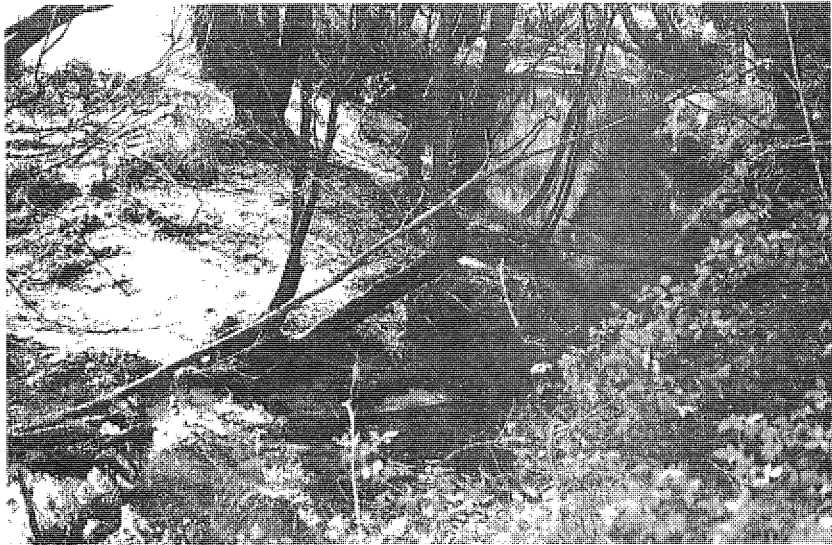
Erosion and subsidence along the Scotsdale Brook. Blackberry is visible in the foreground.
