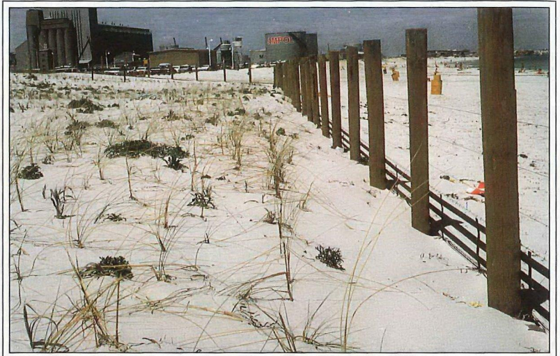
Figure 41. 2 m posts with the first layer (1 m) of Paraweb® attached. The second layer can be attached as the sand has nearly reached the top of the Paraweb®. (photo: J. Broun)
