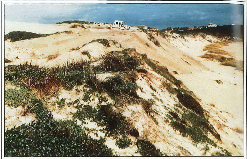
Figure 36. Bulldozing sand dunes to re-form the foredune at Halls Head, Mandurah (photo: J. Broun)
