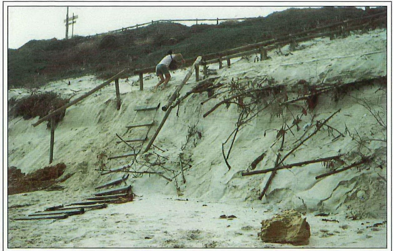
Figure 26. Seasonal undermining of recreational facilities and dune protection works can be severe (photo: J. Brown)
