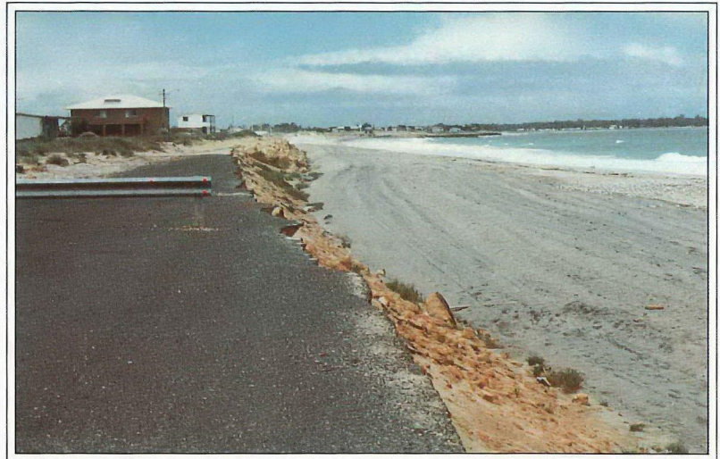
Figure 27 Long-term wave erosion has eroded Ormsby Terrace, Mandurah, threatening houses. This problem was resolved by relocating the road and constructing a series of groynes along the beach (photo: J. Broun)
