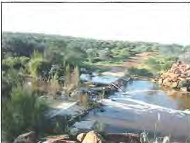
Photograph 3: The old Port Gregory Road crossing although slowly eroding away is still obstructing small to medium flows
