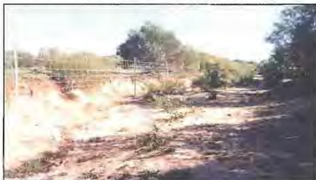
Photograph 14: Fence too close to the floodway which was not protected from washouts in large flows
