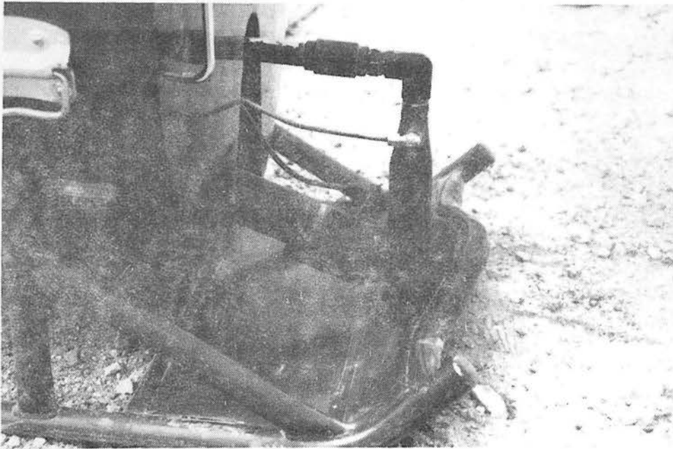
FIGURE 3. BURNER NOZZLE AREA.
