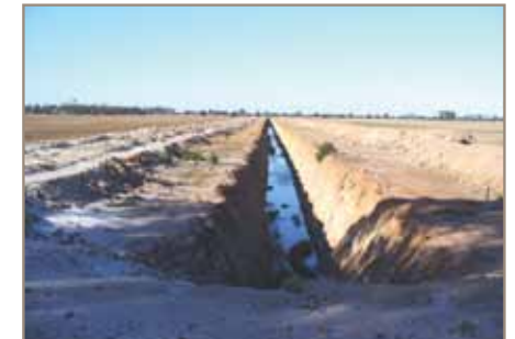
It is estimated that at least 4,000 kilometres of deep open drains have been constructed in the Wheatbelt. Photo – John Lizamore/DEC Esperance
