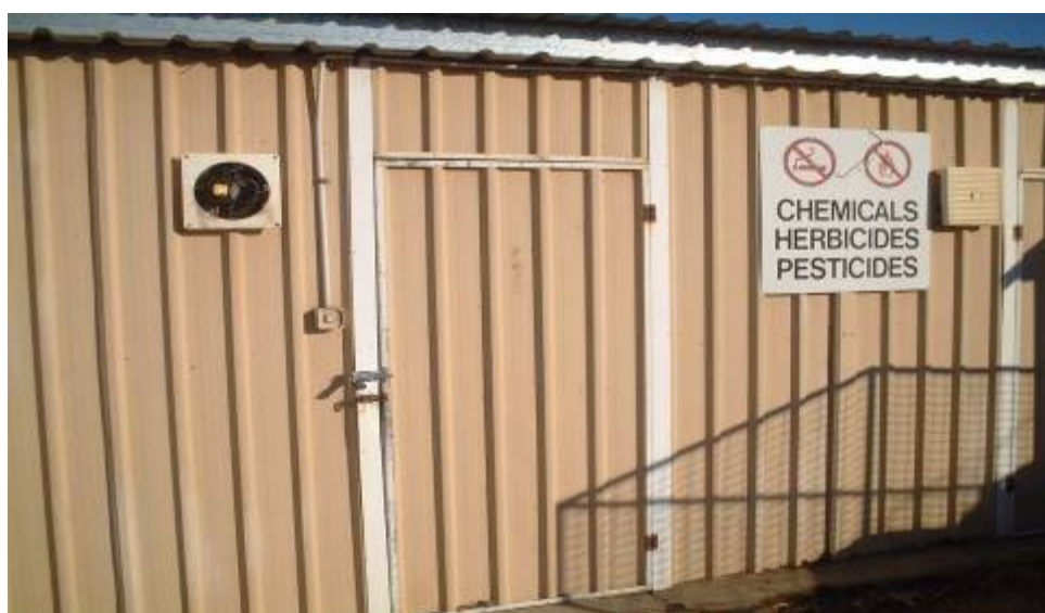
Figure 34: Chemical storage with signage and ventilation (Source: City of Manduarah)
