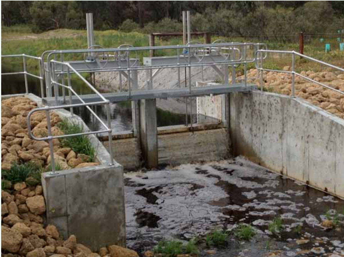
Figure 9. The adjustable height weir, receiving flows diverted from the Mealup Main Drain. Photo – H Bucktin/DEC.
