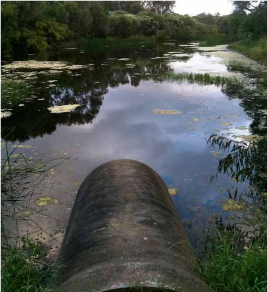
Figure 22. Requirements regarding the placement of stormwater infrastructure in and near wetlands is outlined in the Decision process for stormwater management in WA . Photo – J Lawn.
